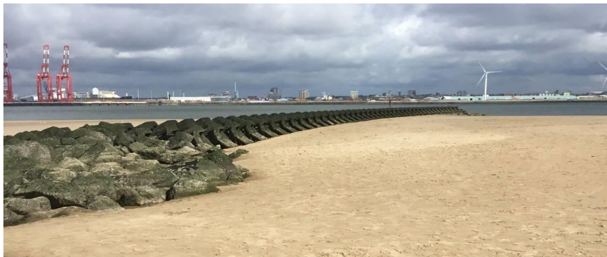
Figure 15: The shore-connected ‘reef-block’ breakwater with a rock stem at Fort Perch. (Photo Source: CH2M site visit 1 st September 2017)
