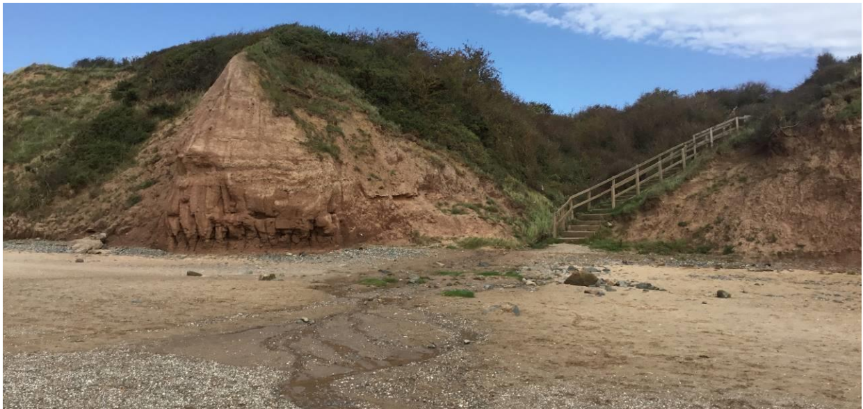
Figure 2: Un defended cliffs at Wirral Country Park (Photo Source: CH2M Site Visit 3 rd October 2017)
