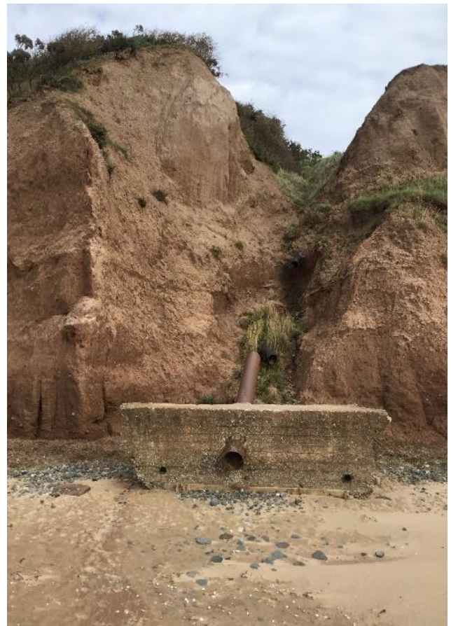
Figure 1: Eroding cliffs at Wirral Country Park, Dee Estuary Coast. (Photo Source: CH2M Site Visit 3 rd October 2017)
