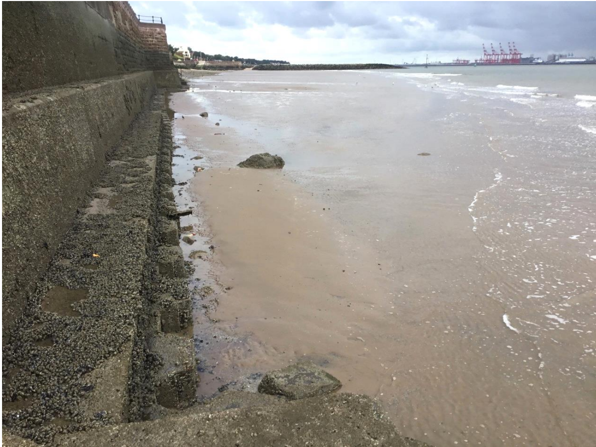
Figure 16: Low beach levels exposing sheet piling at the base of the seawall opposite Wilson Road, between Egremont Groyne and Seacombe Ferry (Photo Source: CH2M site visit 1 st September 2017).
